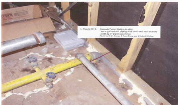
4. Ramada Station to-date: Shows inside galvanized piping going either to dead-ends or inserting pipes into other pipes.
