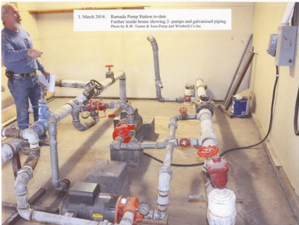
3. Ramada Station to-date: Inside house showing 2-pumps and galvanized piping with valves.
