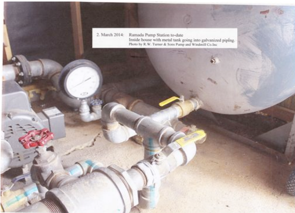
2. Ramada Station to-date: Inside housing with metal tank going into galvanized piping.
